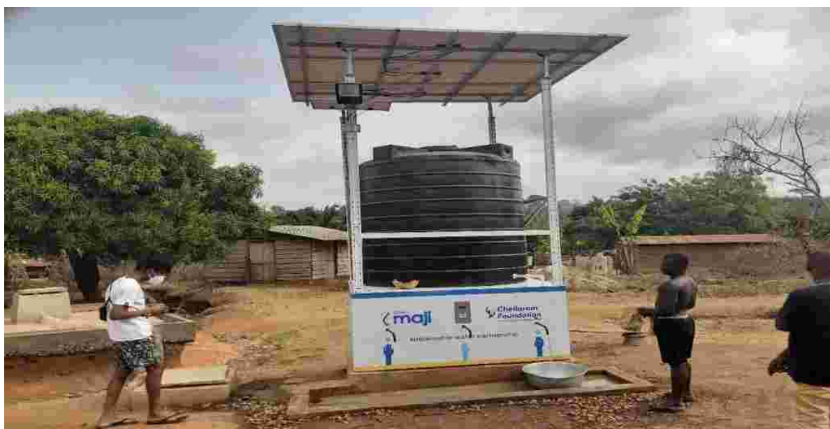
Solar-powered Prepaid Mechanized Borehole at Nseinua Community
